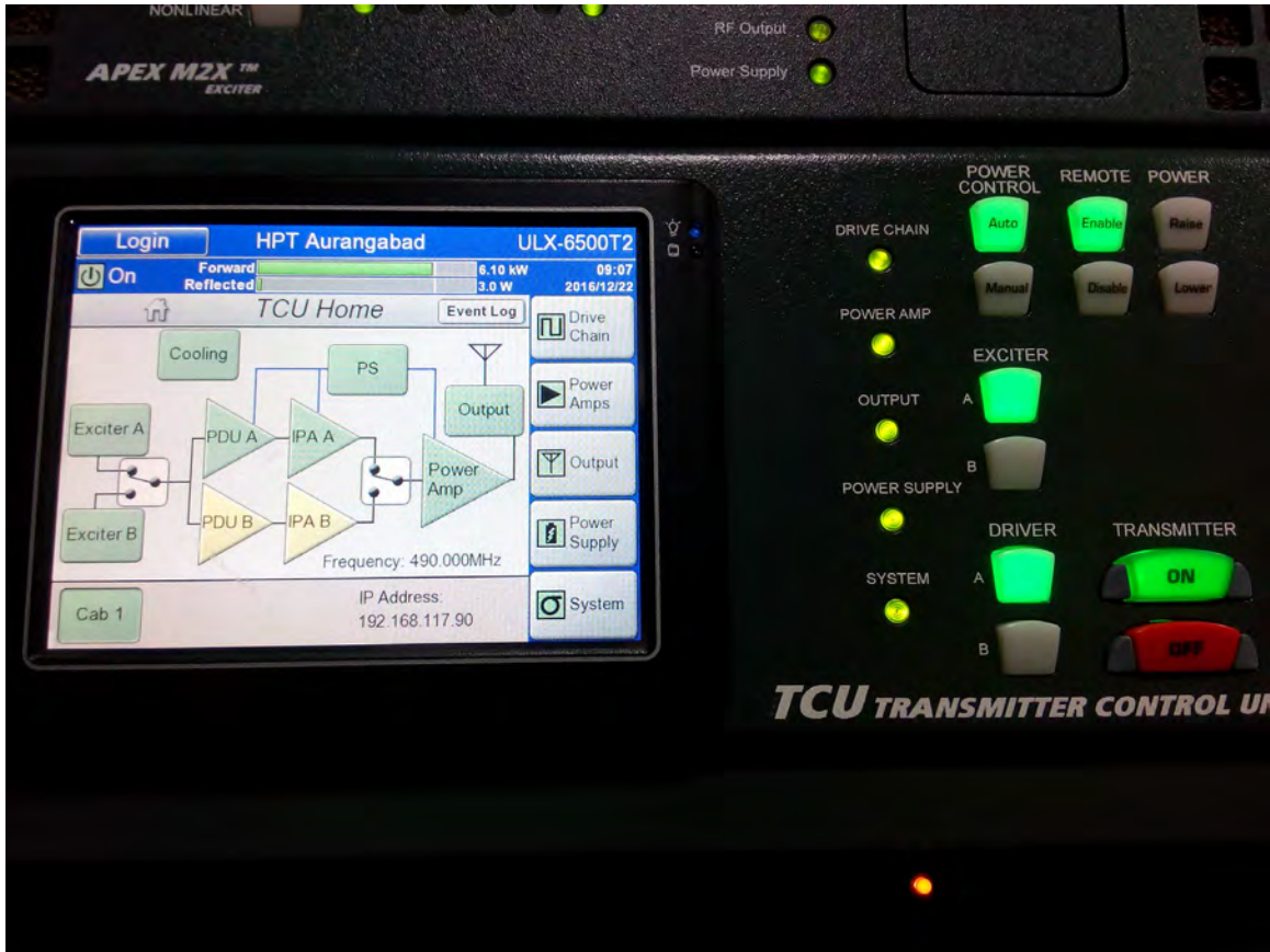
Transmitter Control Unit
