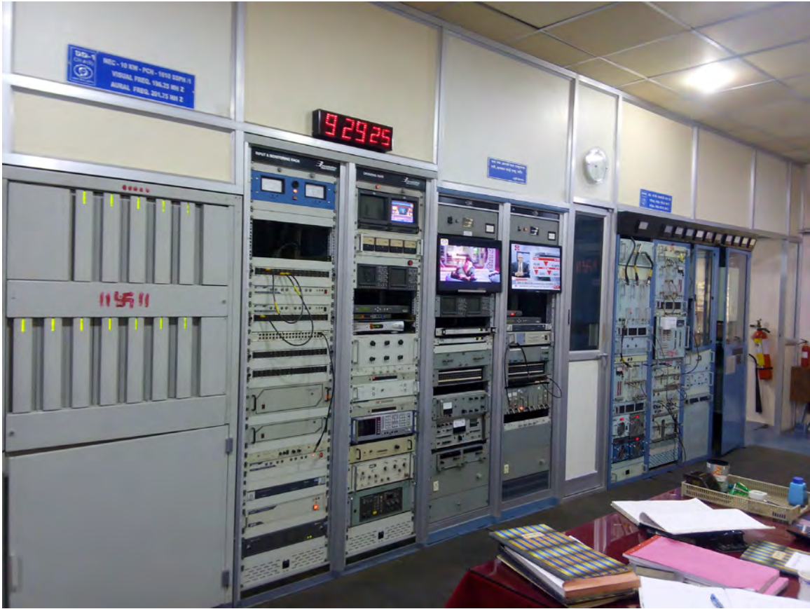
TV Transmitter Hall, HPT(TV) Aurangabad
