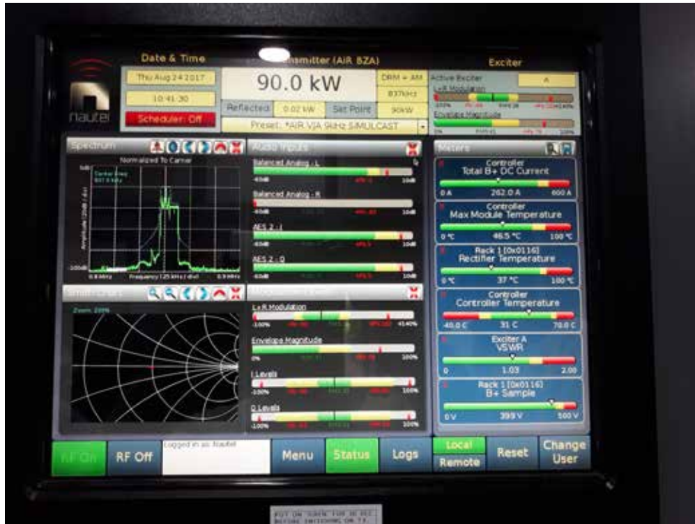
Transmitter Control Unit
