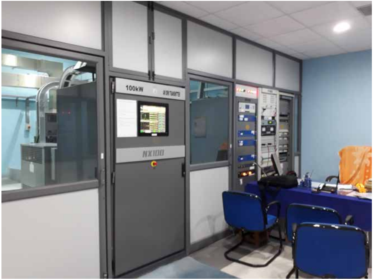
TV Transmitter Hall, HPT(AIR) Vijayawada
